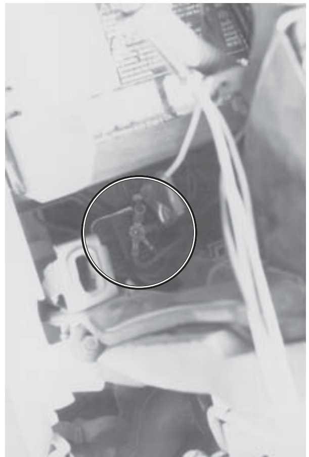
Power Terminal Connection (Adjacent to Battery)
